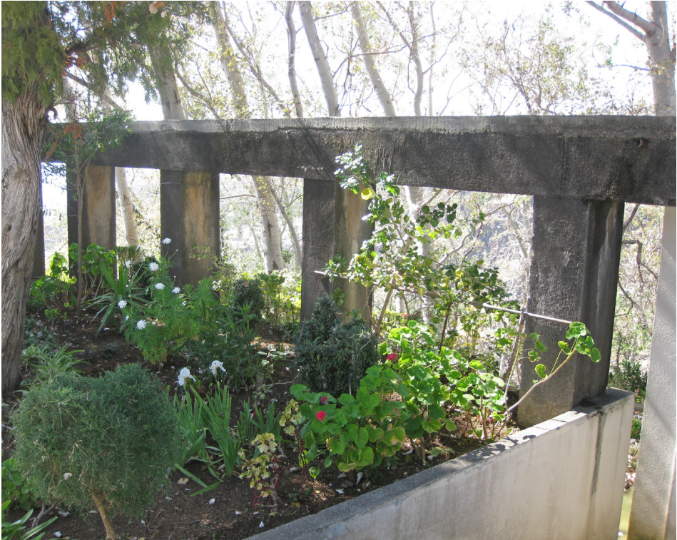
Figure 19. The bridge aqueduct along the west side of the praça at Lombada, with its concrete channel and piers.
