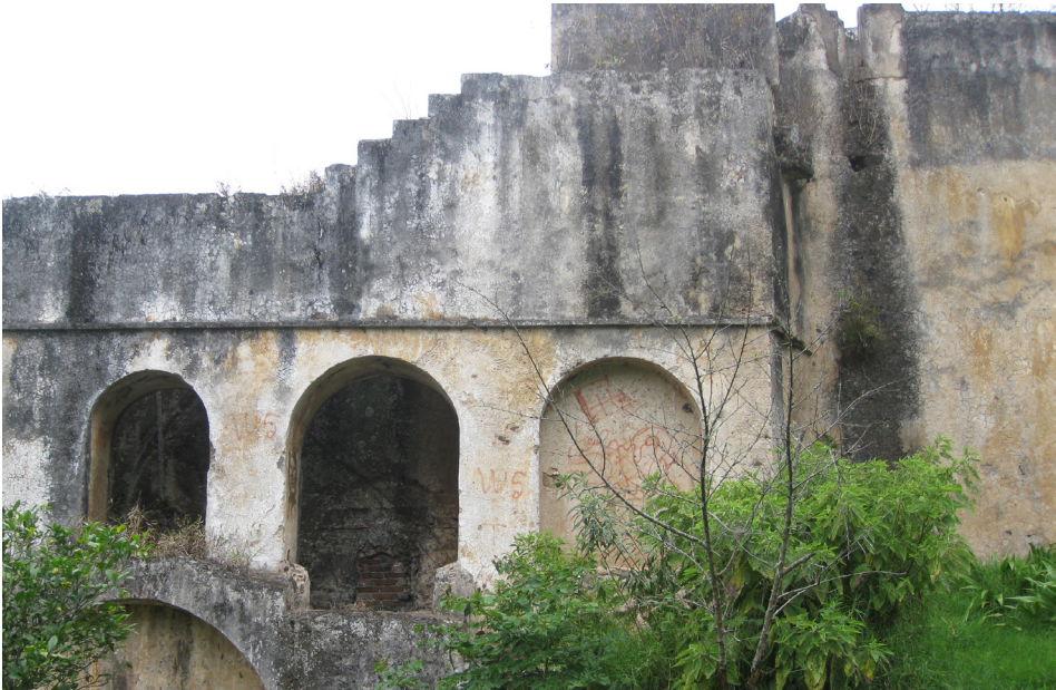
Figure 3. Profile view of the mill structure at Hacienda de Pacho. Water entered the mill through a channel in the upper right, dropped into a penstock behind the arch on the right, and turned a milling device below. Water exited the mill via a chase behind the lowest arch visible in the lower left.
