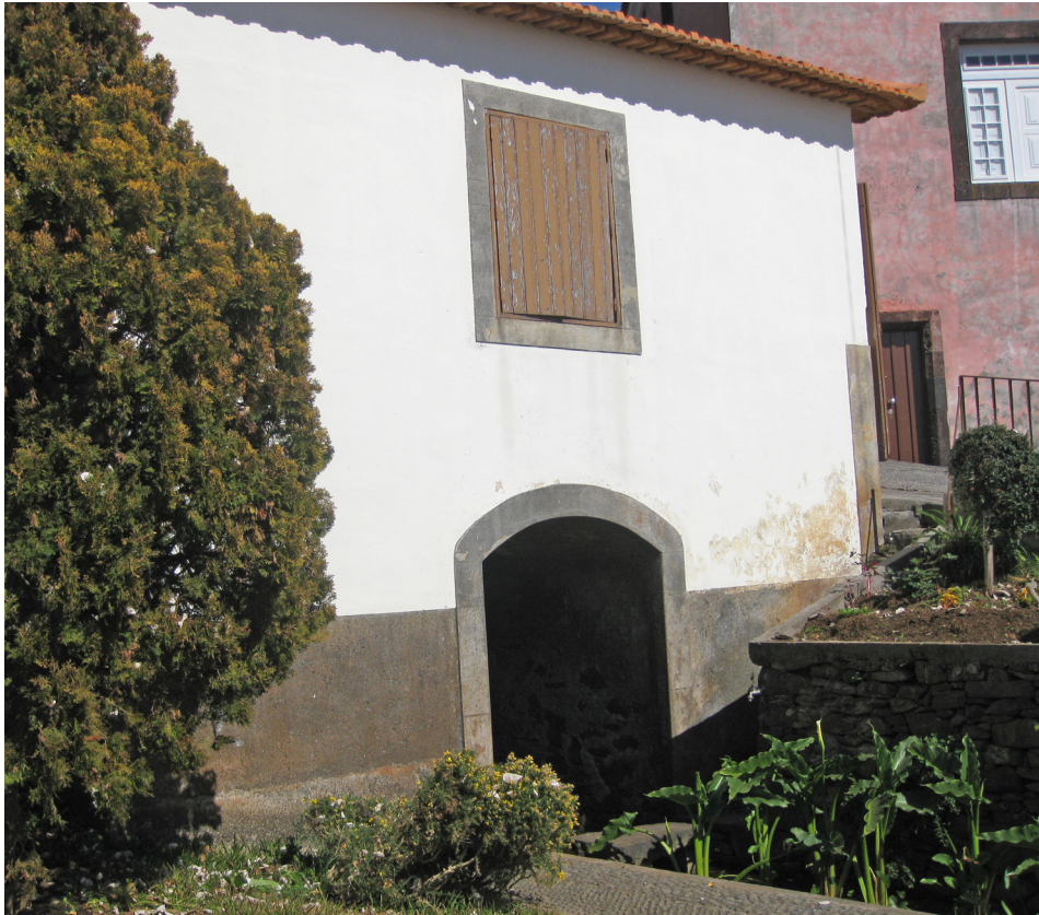
Figure 17. The downslope side of the mill structure at Lombada, Madeira. Evident are the chase below (compare with Figure 8) and the shuttered window on the second level where the millstones are located.
