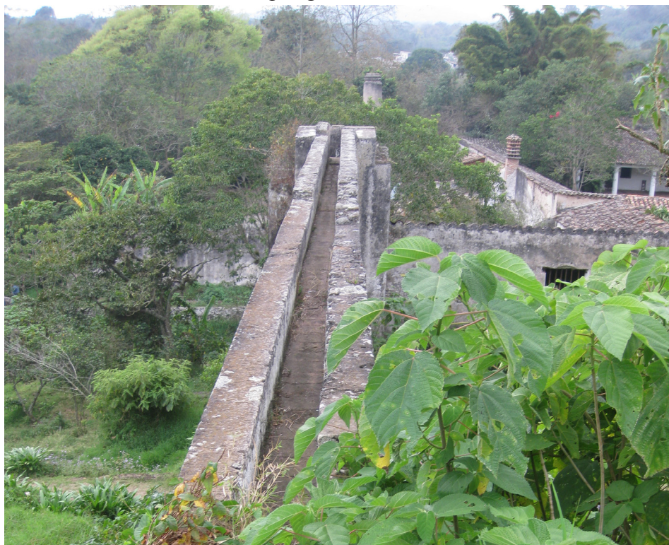
Figure 4. View along the top of the aqueduct that carried water from the spring to the mill
